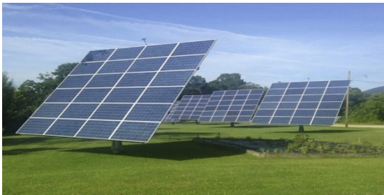
Fig. 1. A solar panel array using the photovoltaic principle [14]
