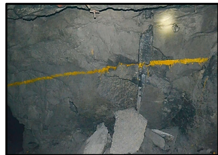
Fig. 9. Pillar compromised by existence of dykes.
