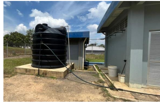
Fig. 2b. The existing building for rainwater harvesting and existing water tank of the groundwater system.
